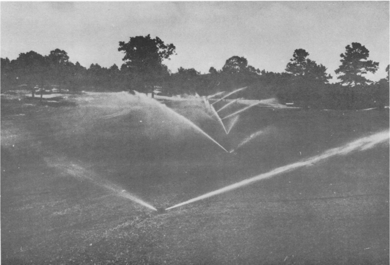
Figure 16-1. A permanent irrigation system in operation.
